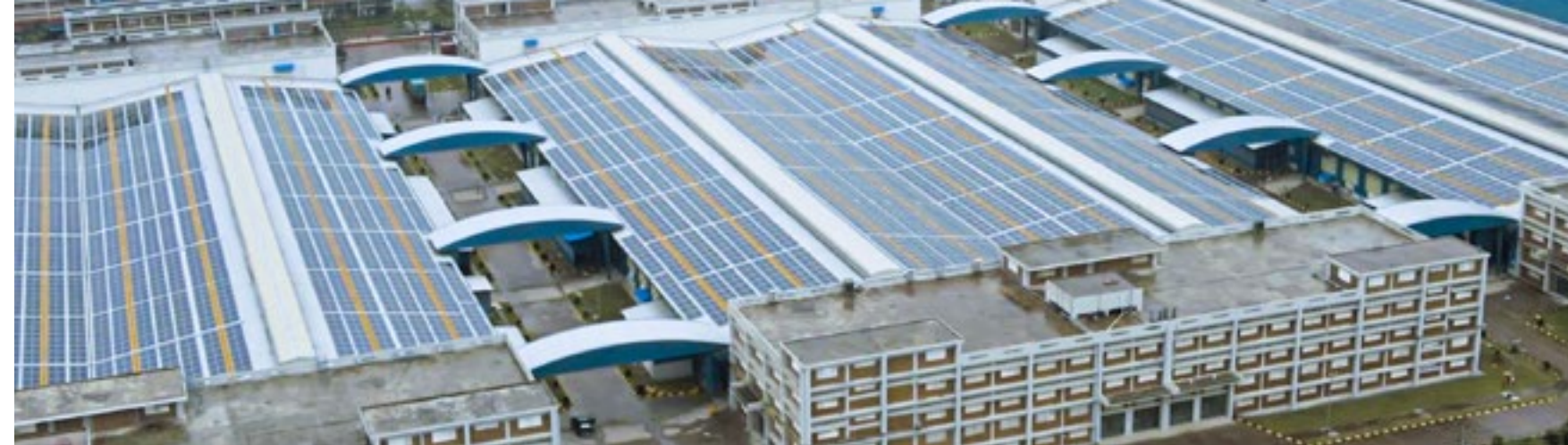
This solar installation in Chattogram, Bangladesh, produces electricity for one of our production partners there. With an output of 16 MWp, enough power is generated to run several textile factories. Any surplus electricity is fed into the public grid.
